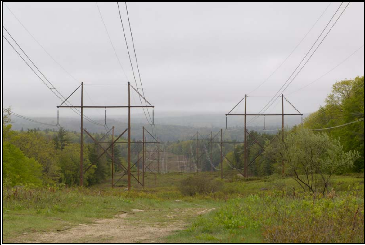
HVAC Power Line Corridor in Deerfield
